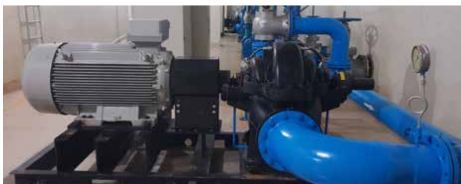
NR. 2 SKDZ-4P 200-630 400kW VIETNAM HYDRAULIC POWER STATION
