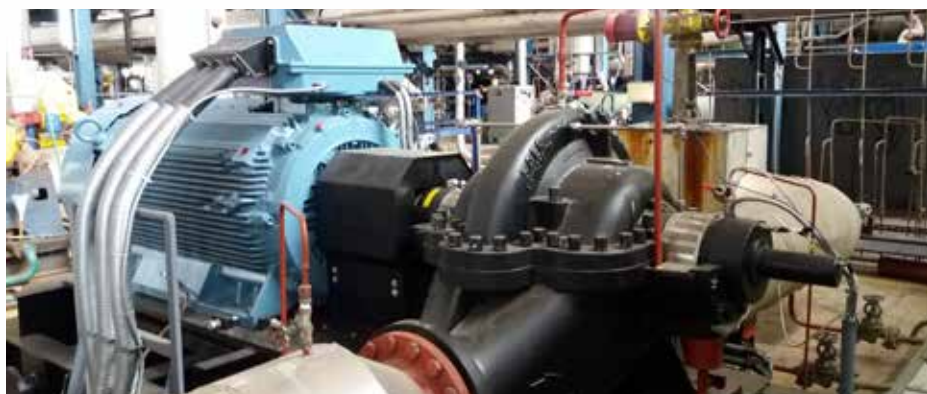
NR. 2 SKDZ-4P 250-750 1000kW SERBIA DISTRICT HEATING
