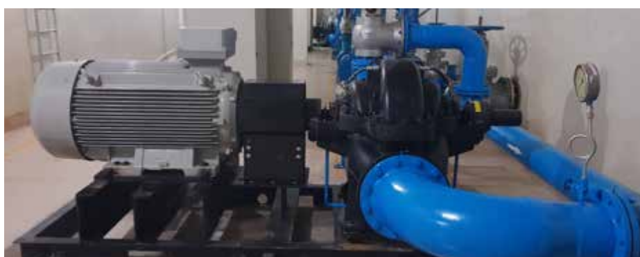
NR. 2 SKDZ-4P 200-630 400kW VIETNAM HYDRAULIC POWER STATION
