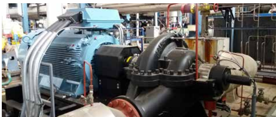
NR. 2 SKDZ-4P 250-750 1000kW SERBIA DISTRICT HEATING
